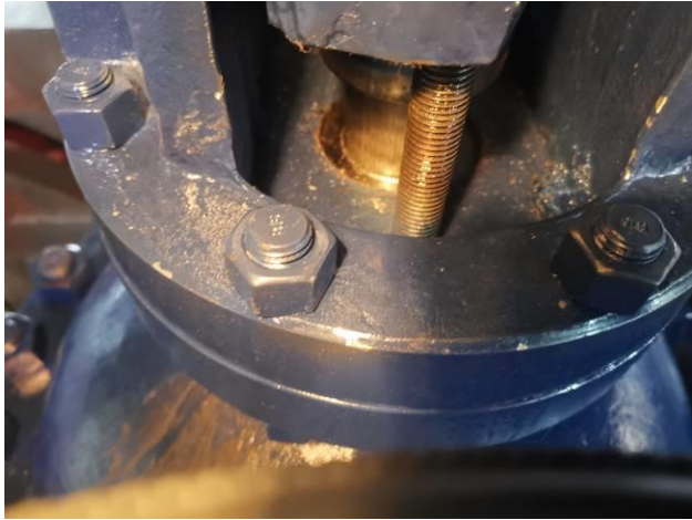
15. Backseat without leakage during high pressure test for Z961Y-63I DN500 Welded Wedged Gate Valve
