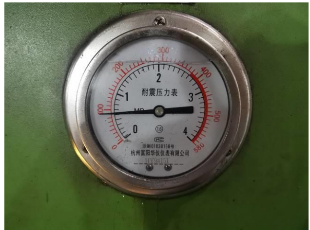
38. Seat test low pressure indicated for Z961H-16C DN900 Welded Wedged Gate Valve
